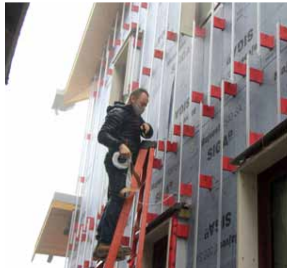
Steve Warrender patches leaks in the air barrier identified by smoke leaks during the blower door test.
