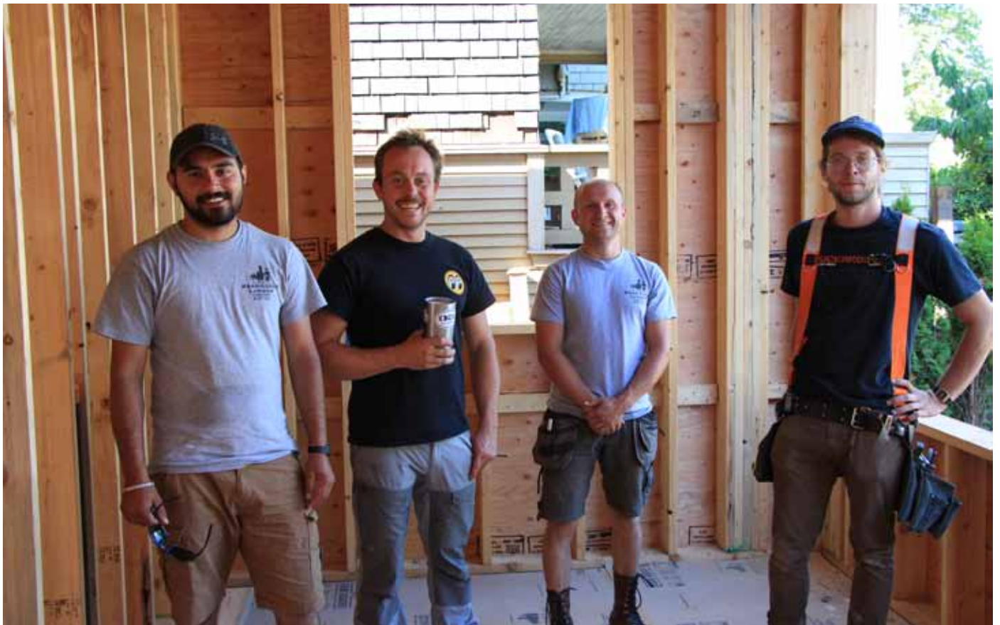
The Kingdom Builders crew: Himmat Gill, Steve Warrender, Max Kazakoff and Matt Burns
